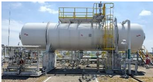
Gambar 2 Neutralizing Backwash Drum
