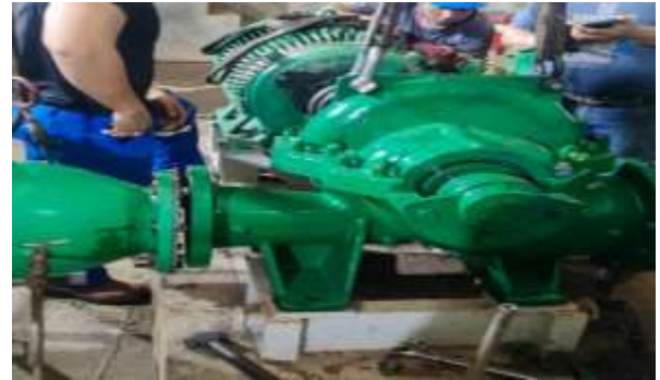
Gambar 2. Pompa Air Intake A
