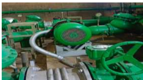
Gambar 3. Feed Water Booster Pump Kondisi Operasional
