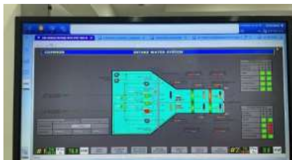
Gambar 4 Memonitor Kinerja Feed Water Booster Pump
